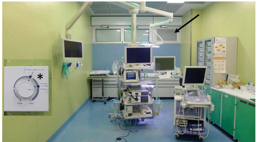
► Fig. 2 Endoscopy room with a dedicated ventilation system (black arrow) to guarantee a negative pressure (asterisk).
