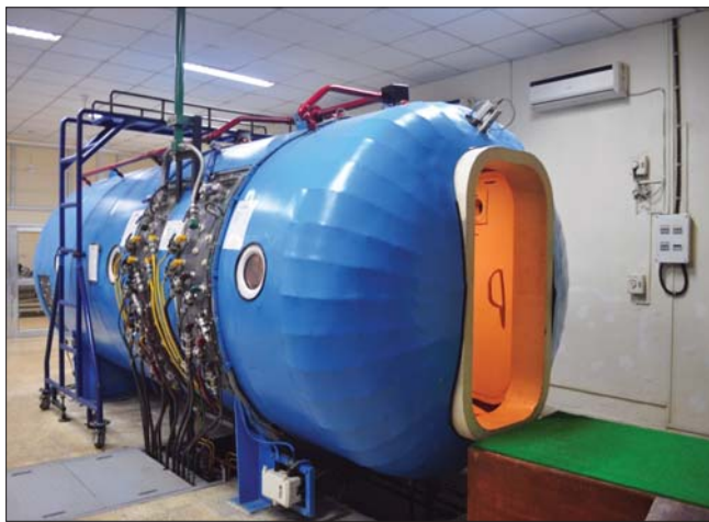
Figure 3: A multiplace hyperbaric chamber installed at INHS Asvini
