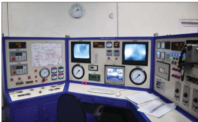
Figure 5: Control panel of the same hyperbaric chamber
